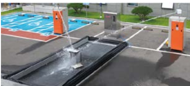
3. The deployment of a fire extinguishing water tank
